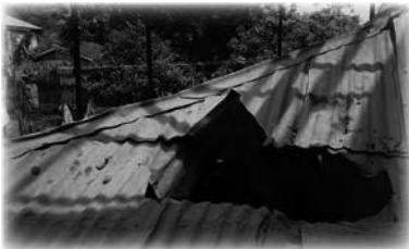
The Roof that was Pierced by the Large Piece of Rock
